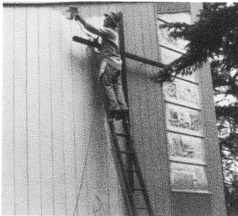
The new Girdwood church, built with earthquake relief money, was later moved to a new site. Here a volunteer worker is painting the building.
